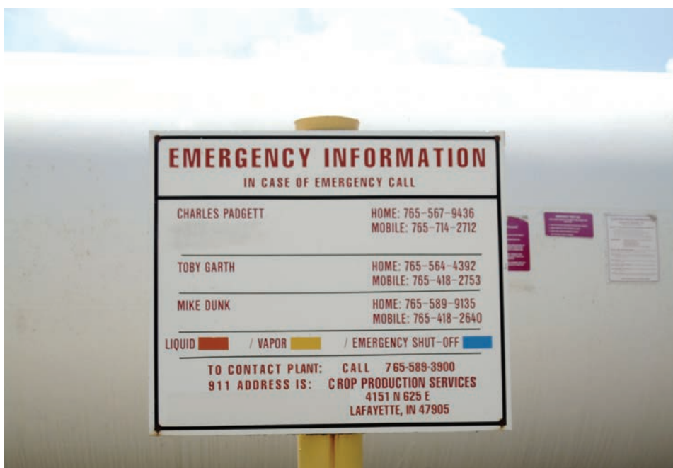
Emergency information is often present at the bulk storage tank as well as the main entrance.
